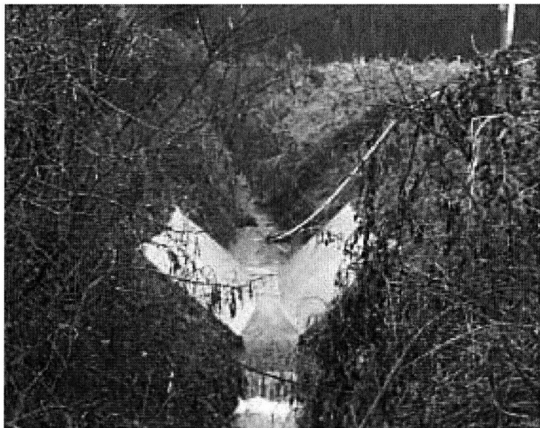
Fig. n° 2 : Pre-formed flume structure imbedded in the ditch at site A1
