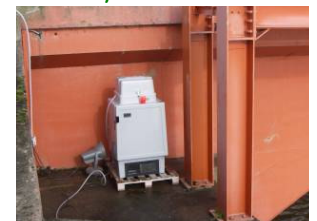
Automatic flow-triggered water sampler at Arzal reservoir
