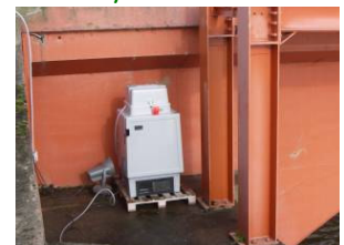
Automatic flow-triggered water sampler at Arzal reservoir
