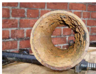
Figure 2: A cut of a segment of pipe to show incrustation
