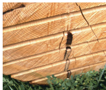
40. The absence of pruning leaves knots that decrease the timber quality (here: a branch that created a non-adherent knot in the most external planks).
