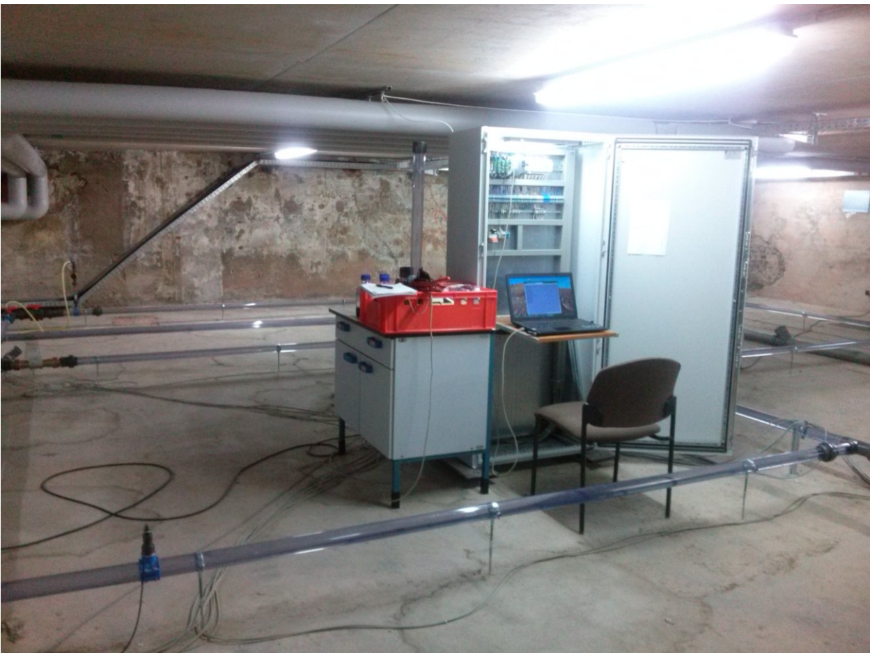
Figure 5: "Control room (SCADA System)" of the test network
