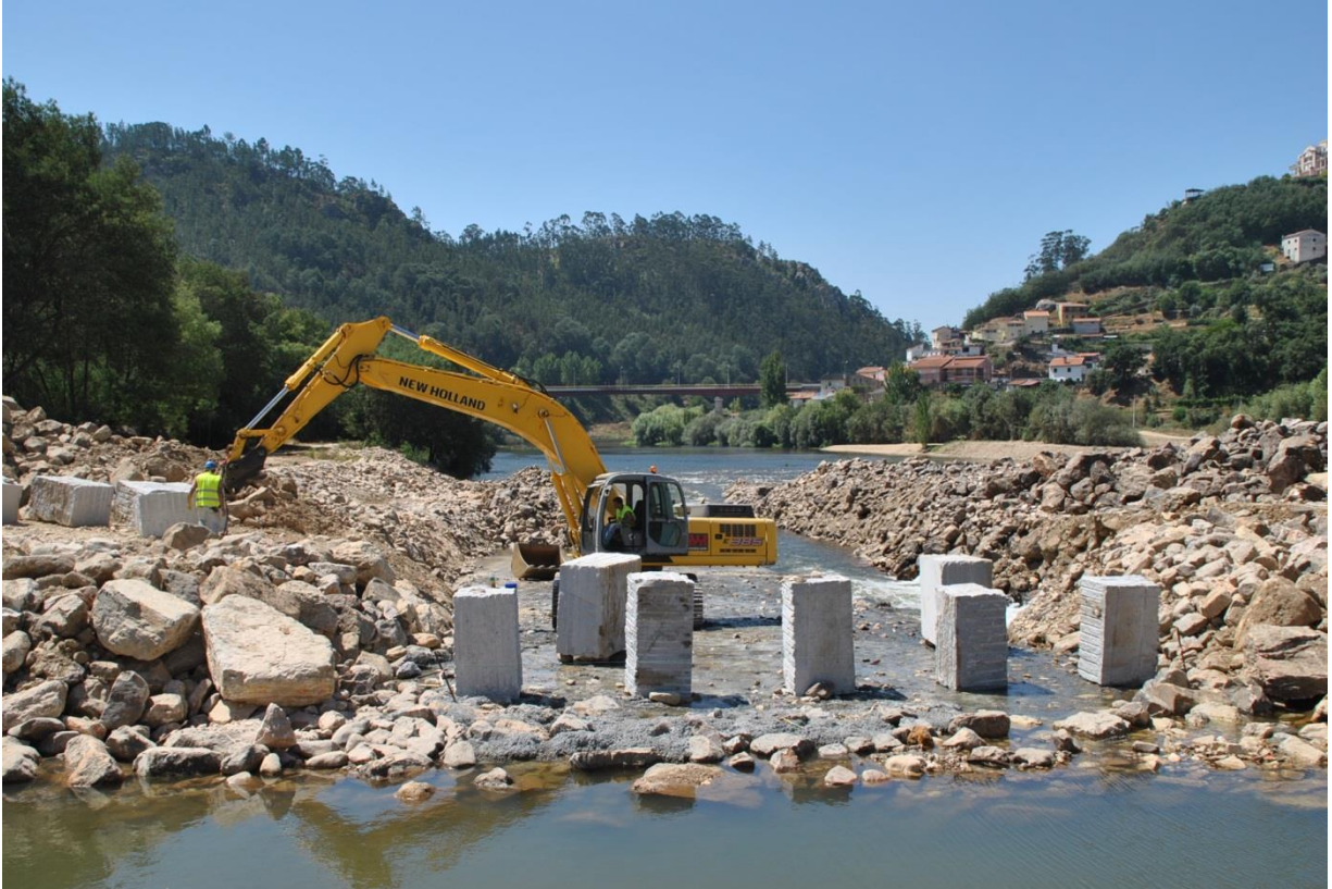
Figure 4.19. Construction of a nature-like fish passage in River Mondego (Penacova weir, July 2015) (Photo: Pedro R. Almeida).
