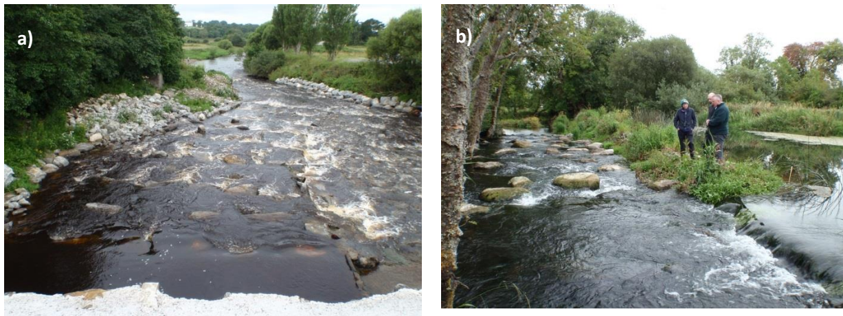
Figure 4.21. Rock ramps installed in a) Abbeyfeale, Feale catchment. Feale is a salmon and sea lamprey catchment under Habitats Directive, and b) King's River, Nore catchment.
