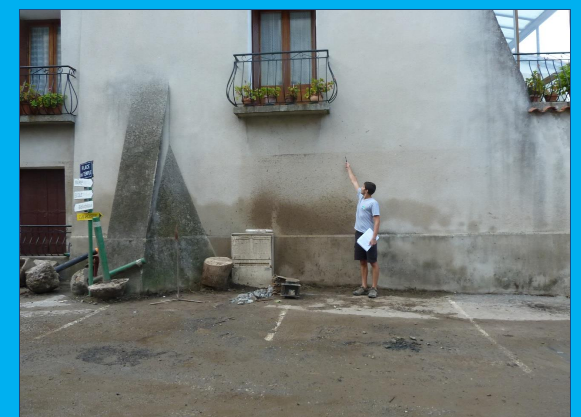
Witness mark of the flood of September 19-20, 2014, in Saint-Laurent-le-Minier (Hérault) - Source : C. Saint-Martin (Irstea, 2015)
