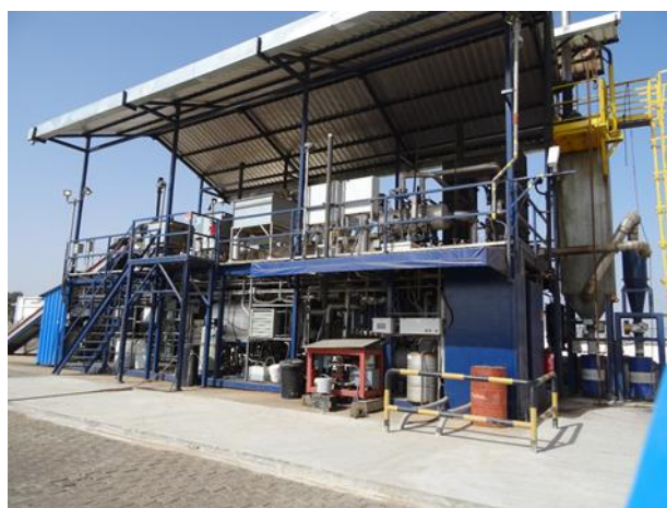
Figure 17 Omniprocessor installé sur la station de Pikine
