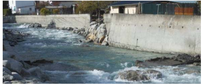
FIGURE 7 - RUPTURE ET REPARATION D'URGENCE D'UNE DIGUE - GAVE DE CAUTERETS - PIERREFITTE (65) - 2013 (ONF-RTM)
