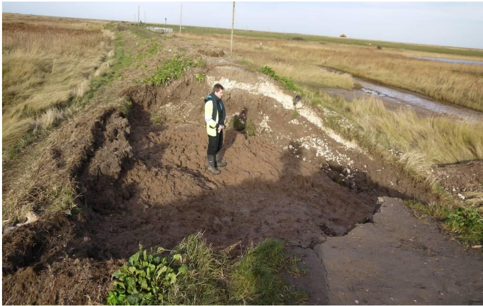
Figure E-1 Damage to levee at Cley, North
