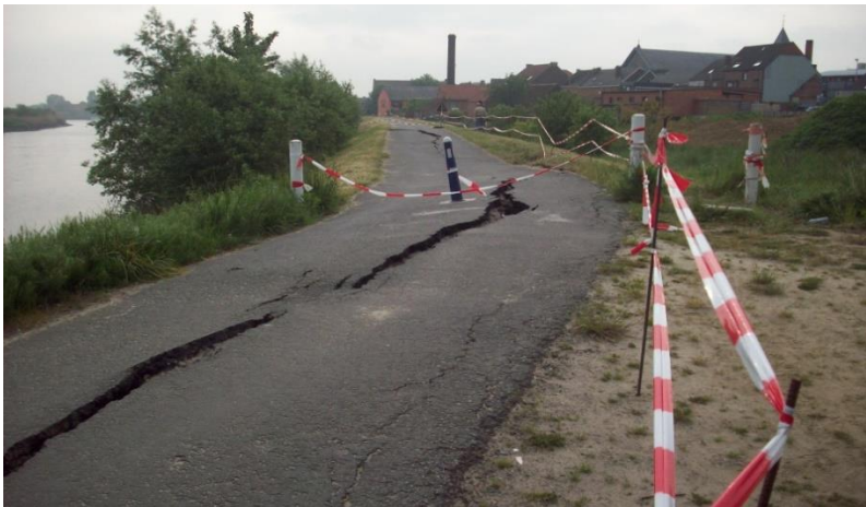
Figure B-13. Slope instability in Schoonaarde along the Schelde (Source: De Vlaamse Waterweg nv)
