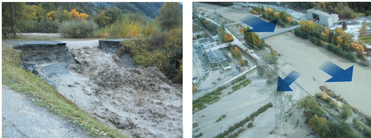
Figure CH-9 (left): Levee breach at the River Rhone near Chamoson in October 2000 [021].
