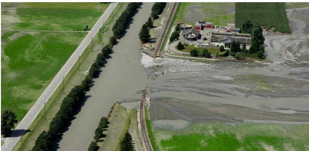
Figure CH-11: Levee breach at river Aare near Meiringen (BE), August 2005 (© Swiss Airforce).
