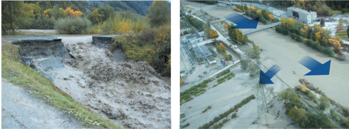
Figure CH-9 (left): Levee breach at the River Rhone near Chamoson in October 2000 [021]. Figure CH-10 (right): Water outflow after levee breach near Chamoson in October 2000 [021].
