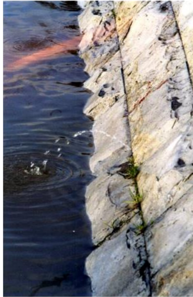
Figure F-6: Post flood inspection finding evidence of leakage in the masonry revetment, probably involving an important void behind the revetment, filled with water during the flood (source: Rémy Tourment)
