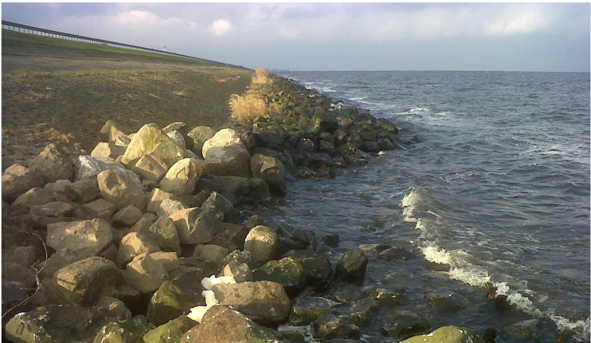
Figure NL-3: Relatively limited damage due to collision of large ship. Note that most of the levee slope has either stone or asphalt revetment, with grass only near the crest
