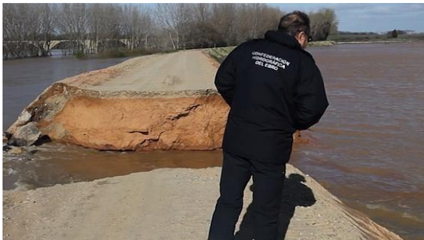
Figure ES-6. Example of partial failure in a levee due to an inadequate foundation.
