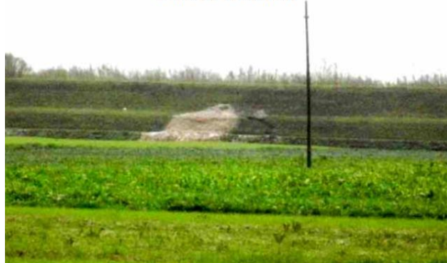
Figure IT-8: Breach initiation along the Secchio River in 2009.
