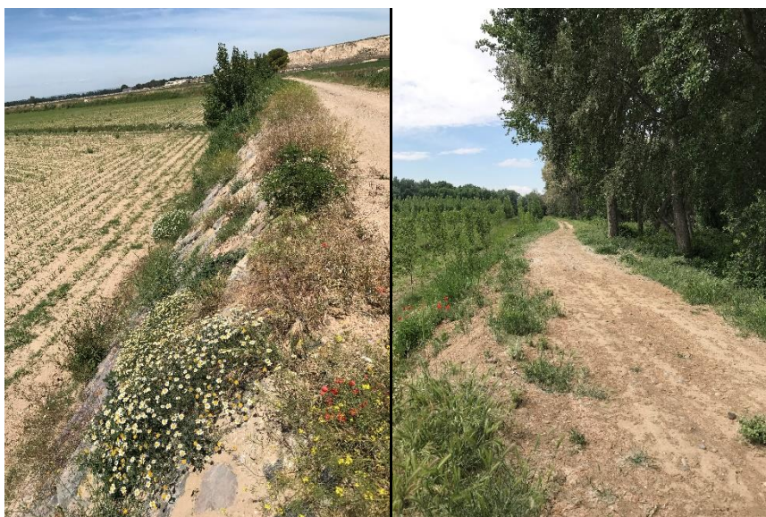
Figure ES3a: Levee segment in the Ebro river in Torres de Berrellen (Zaragoza). Source: MITECO (Spanish Ministry for Ecological Transition), and, Figure ES3b: Levee segment in the Ebro river in Pradilla (Zaragoza). Source: MITECO (Spanish Ministry for Ecological Transition).
