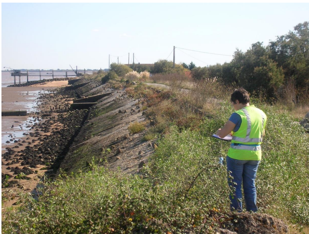
Figure F-5: initial inspection on an estuarine levee in Gironde (source: Rémy Tourment)
