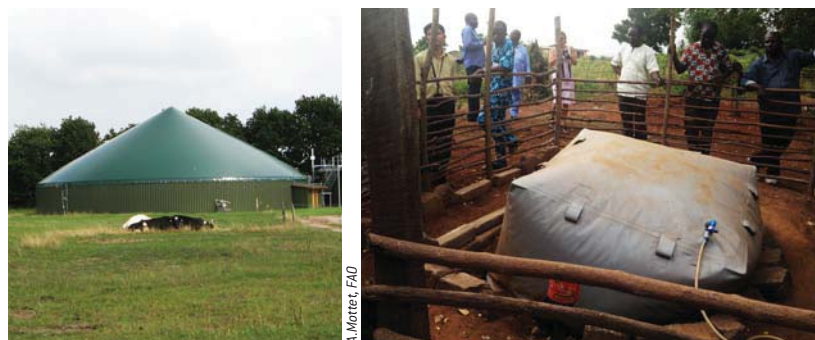
These methanisation plants (in Germany, left, and in Ghana, right), considerably different in size, both produce renewable energy (biogas) from livestock manure.
