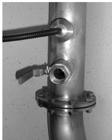
Figure 2. TENferm measuring head mounted in a pipe (top), sampling valve (below)
