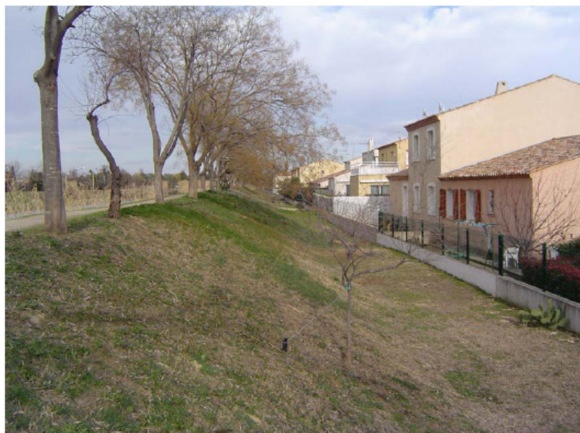
Figure 10: Recent housing too close to the dike, in Lattes (source: MEDD, 2006)
