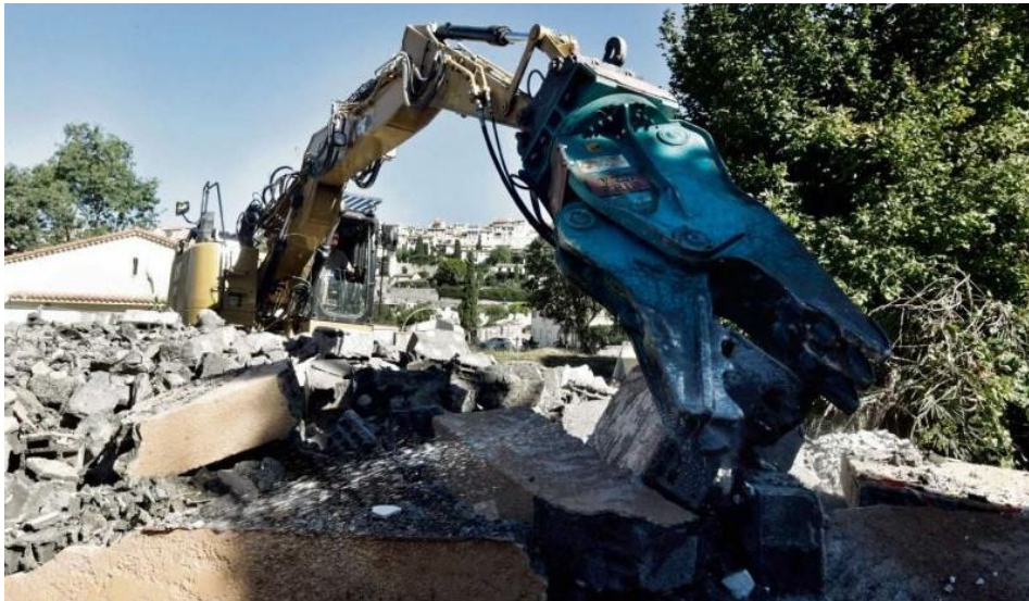
Figure 56 : Removing houses located in the Brague high flood risk area has yet started (source: Nice-Matin, © Frantz Bouton, https://nouveau.pressedd.fr , published on Oct. 3 rd , 2018).
