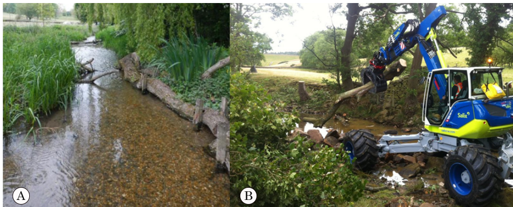
FIGURE 1.2. (a) LW used in a restoration on the lowland River Gade, UK (Grabowski et al., 2019). (b) Installing LW for the restoration on River Washburn (source: https://www.salixrw.com/solution/river-washburn-river-restoration/ ).
