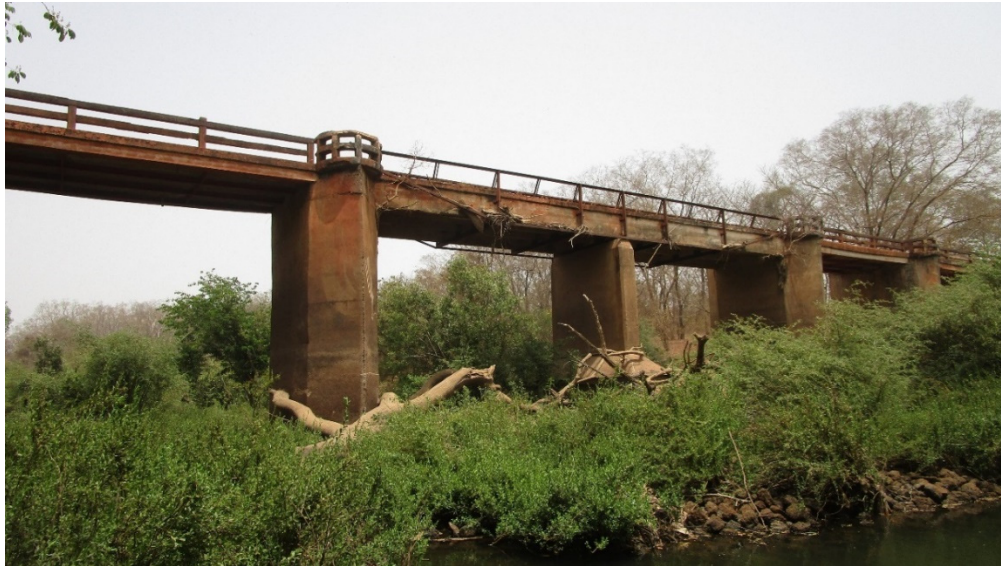
Figure 15. Bridge of the Koundara-Youkounkoun road, northern Guinea, on the Koulountou River. Built in the 1950s, it was flooded by the streamflow in August 2018, depositing whole trees (bottom) and wood debris (on the bridge deck).
