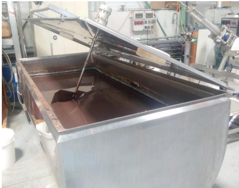
Figure 16: Vinasse storage tank
