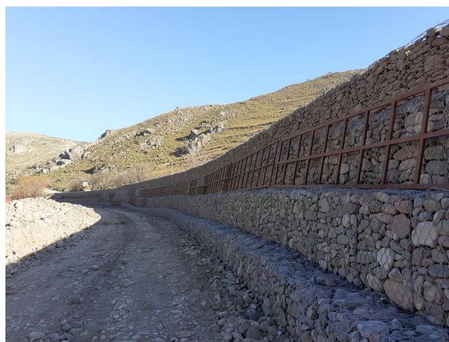
Photo showing the construction "Serazaneti" to stabilize the river bank and to enhance its capacity to accept higher stream power during the flood event (Taken by facebook page "Ο χρούσος")
