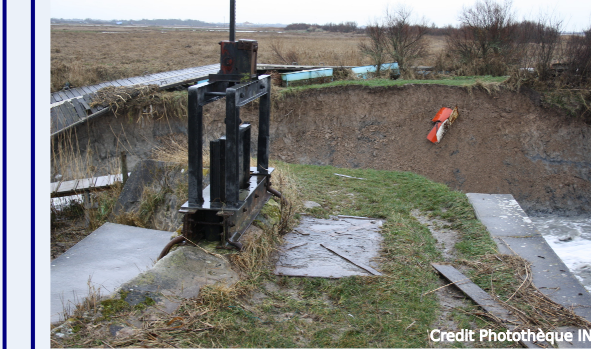
Figure 8: Drainage equipment in Saint Laurent de la Prée
