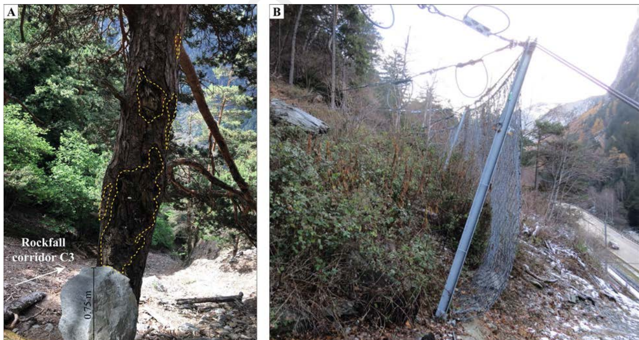
Fig. 3 View of (A) a multi-impacted pine stem (yellow dotted line) sampled at the vicinity of the cliff and (B) rockfall protection barriers installed in the lowest portion of the talus slope
