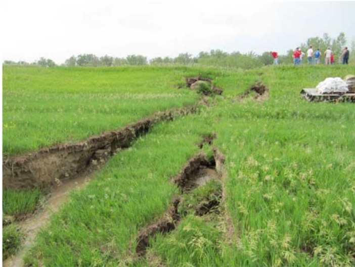
Figure 3.13 The initial distress in the levee L-575.
