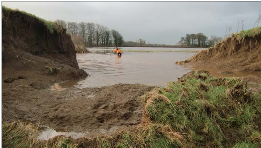
Figure 3.3 Photograph of the breach.
