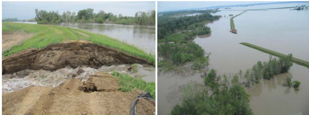
Figure 3.15 The initial breach of the levee L-575 (left), and the levee breach after complete interior flooding (right).
