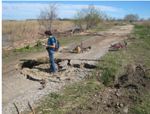
Figure 3.51 Sinkhole on the levee crest (Photograph by Patrice Mériaux).
