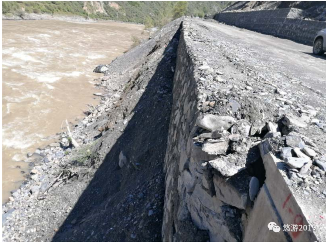
Figure 3.61 Outwards displacement of the bank slope and retaining wall.
