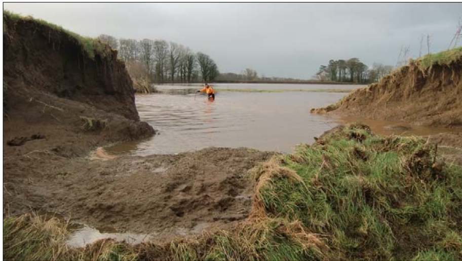
Figure 3.3 Photograph of the breach.
