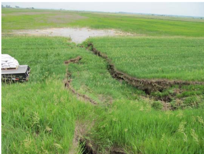
Figure 3.14 Initial distress in levee L-575 showing alluvial fan.
