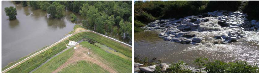
Figure 3.9 Seepage occurring at the toe of the levee prior to breach (taken around 0800 hr, 23 June 2008) (left), and Sand bag effort prior to breach (taken around noon on 26 June 2008) (right).
