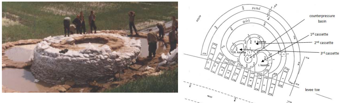
Figure 3.39 Counterpressure basin for related cassettes (left) and location of sand cassettes (right).
