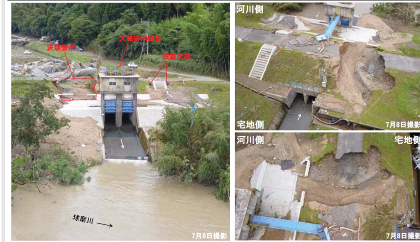
Figure 3.33 Example of overtopping from the presentation 'Picture-Card Show Project' in JGS-JCES', contribution by K. Maeda, M. Ishihara and H. Mori, using materials from the Ministry of Land, Infrastructure, Transport and Tourism in Japan.
