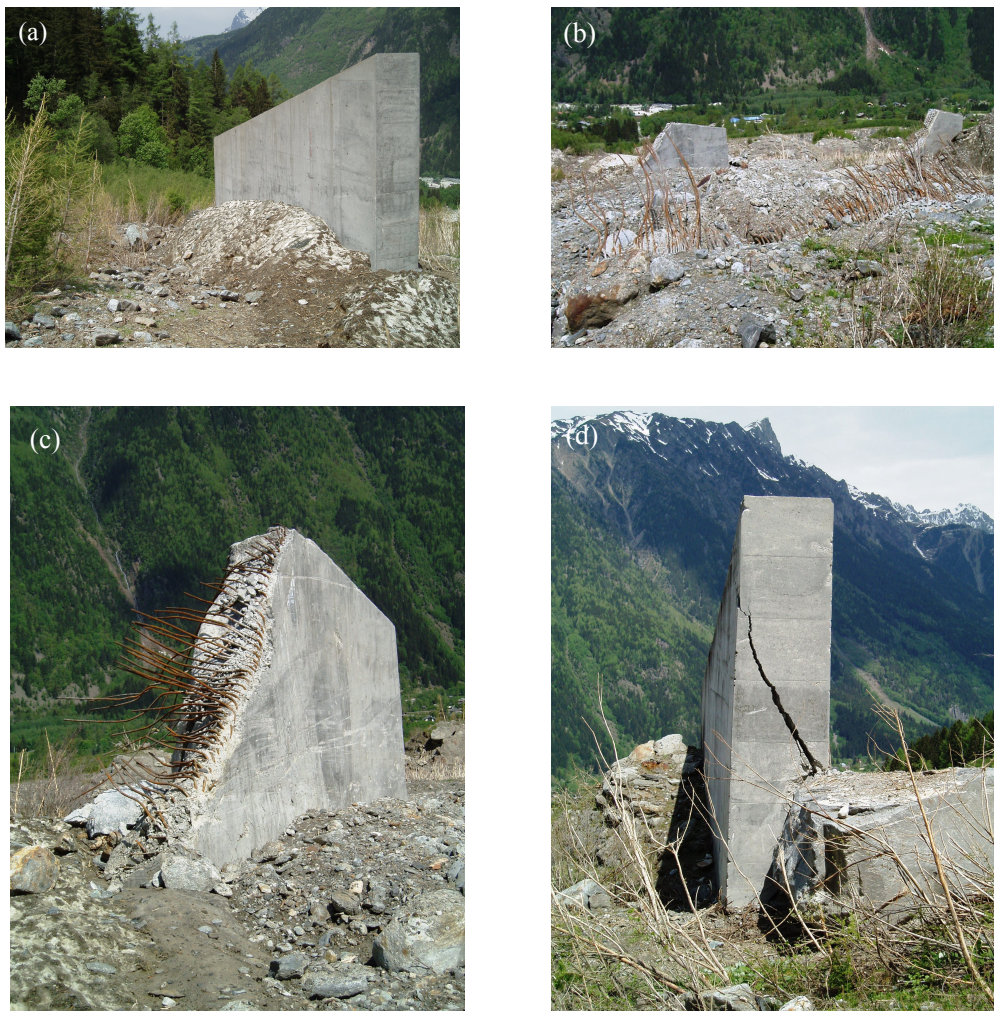
Figure 2: Overview of damage caused by a snow avalanche to different elements of the Taconnaz reinforced concrete structure during the winter of 2005/2006. Damage intensity is sorted in four states: (a) without damage; (b) fully destroyed; (c) partially destroyed; (d) with cracks (Photo credits: ©François Rapin/INRAE).
