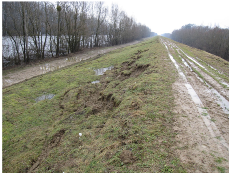
Figure 19. Dyke top structure with rutting caused by traffic and with local erosion failures typical for wet seasons.
