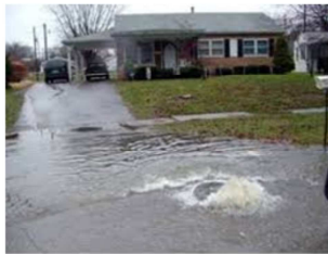
Sanitary sewer manhole overflow
