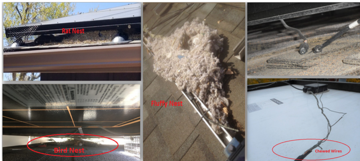
Figure 3. Pest damage to solar PV arrays [25].
