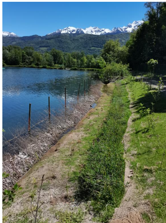
Figure 2. SWB structures using plants of different species and with a strong soil stabilization power thanks to their root development. These works help protect the bank from erosion.
