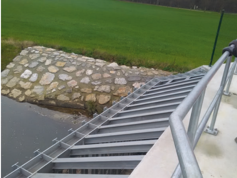
Fig. 15.5 The FreeStation was installed on the driftwood barrier at the lower end of the newly built Brdnikova reservoir
