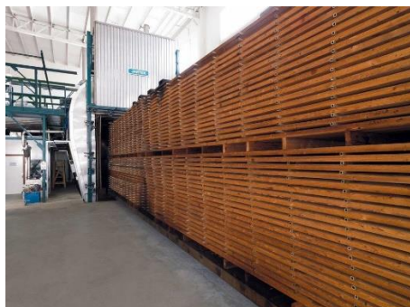
Fig. 3: Thermal modification plant in Mazand Choob Aria Co. based on Thermowood technology
