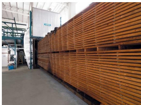
Fig. 3: Thermal modification plant in Mazand Choob Aria Co. based on Thermowood technology
