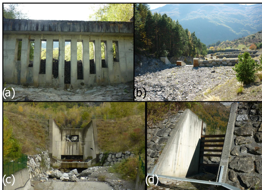
Figure 2. Examples of debris basins used in the analysis: (a) the Lavanchon torrent (Saint-Paul-de-Varces community), (b) Verdarel torrent (Saint-Chaffrey community), (c) Claret torrent (Saint-Julien-Mont-Denis community) and (d) Nant Croex (Ugine community).
