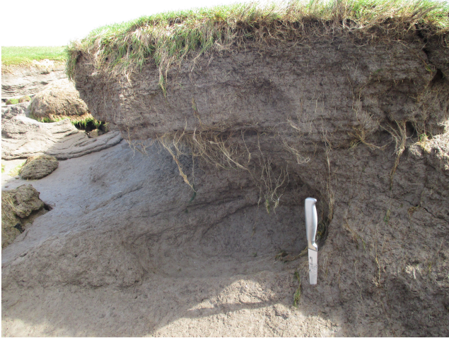
FIGURE 5. Example of undercutting at the base of the cliff, while the upper cliff overhangs and appears to be held in place due to tensile strength provided by the roots. Photo by I. Moeller taken at Warton Marsh, Morecambe Bay (UK) in July 2018. The knife in the photo is approximately 20 cm in length. [Colour figure can be viewed at wileyonlinelibrary.com ]
