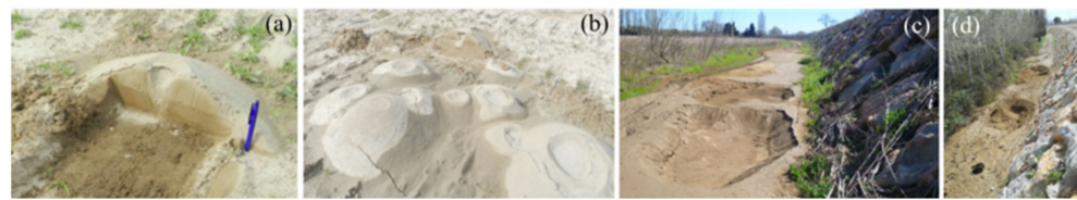
Figure 1. (a,b) Sand boils in the protected area, (c,d) Sinkholes observed around the levee toe.
