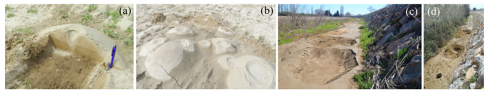
Figure 1. (a,b) Sand boils in the protected area, (c,d) Sinkholes observed around the levee toe.
