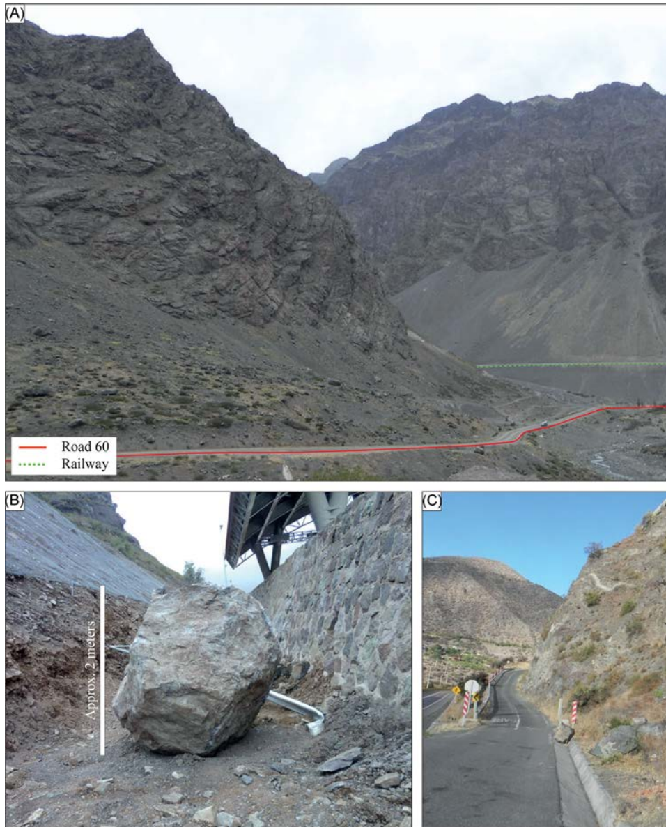
FIGURE 3 (A) Fractured rock cliffs overhanging sections of road No. 60 and Transandine railway ( // INRAE Grenoble). (B) Rockfall event that occurred in 2012 at road No. 60 toll ( // Ministerio de Obras Públicas, Gobierno de Chile). (C) Recent small boulders on the side of road No. 60 (INRAE Grenoble).
