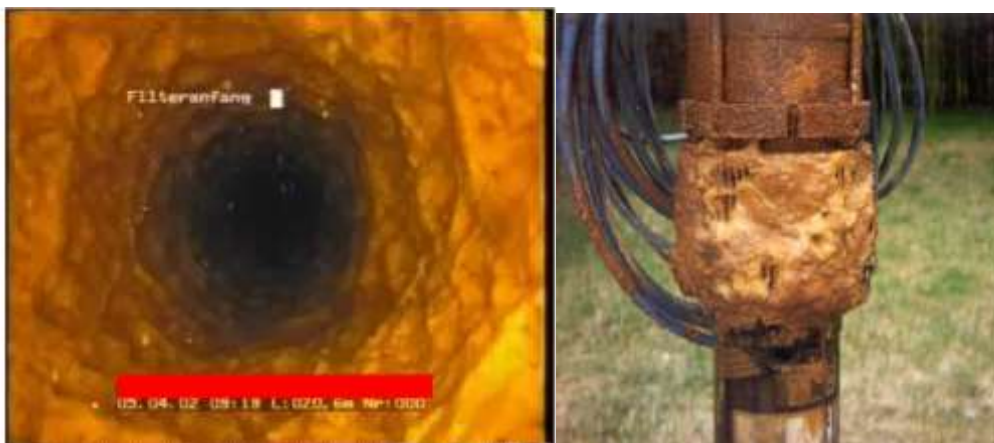
Figure 1: left: clogged well, ochre deposits inside the screen; right: clogged pump, ochre deposits at the pump intake, both ©BWB
