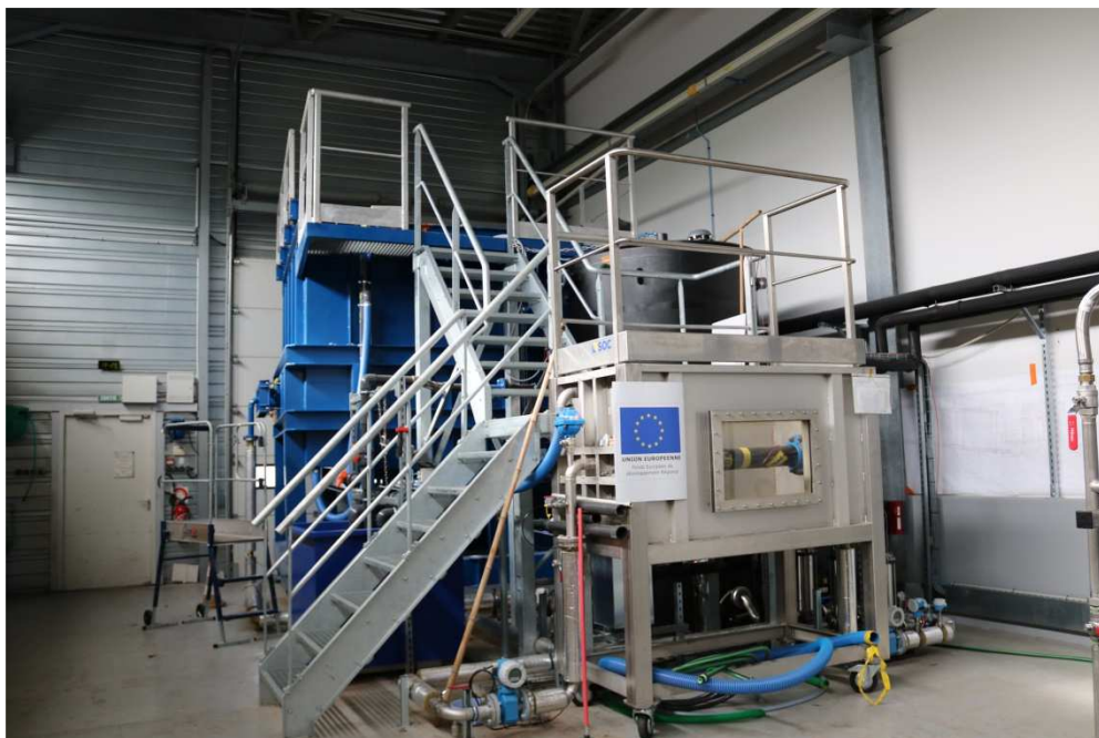
FIGURE 1 : PILOTE FUITE - HALL TECHNIQUE
