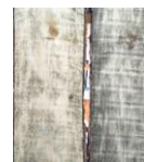
Fig. 12: fungi colonization on the cladding at the craft laboratory, photo by the author.
