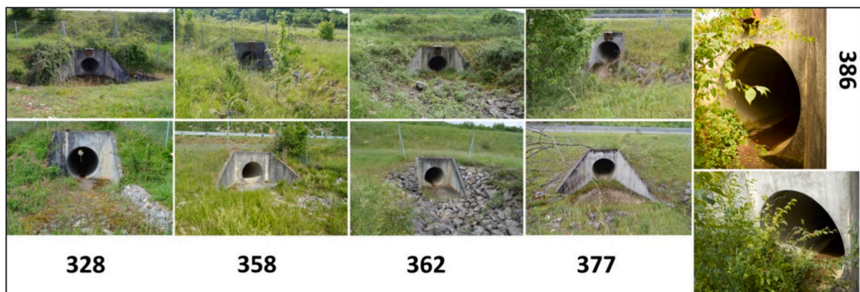
Fig. 2. Overview of the western (top line) and eastern (bottom line) openings of each of the five underpasses studied in the ‘Causses du Quercy’ regional natural park, France. The figures refer to site ID (see Table 1).
