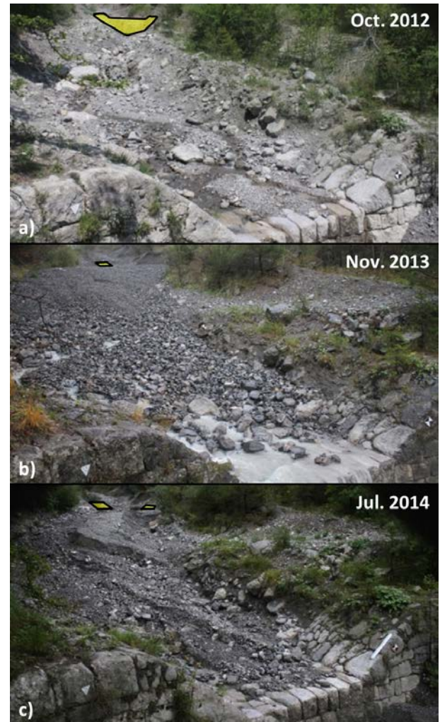
Figure 5.2 – Illustration of slope fluctuations in the vicinity of old check dams in the Manival torrent -Fr. (visible part of the upstream check dam colored in yellow): a) eroded reach with a mild slope in Oct. 2012, b) filled reach with a steeper slope, deposit burying the upstream structure in Nov. 2013 and c) partially eroded deposits in Jul. 2014 (Photos courtesy of C. BEL)
