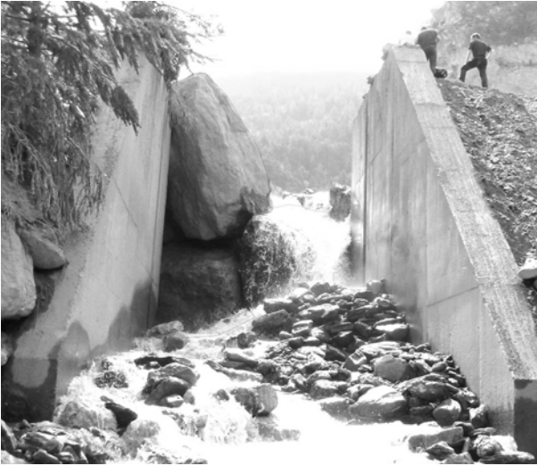
Figure 2.5 – Downstream view of the St Antoine sediment trap after the 31 July 2014 debris flows: mechanical blockage of the 5-m-wide, 8-m-high slit dam by three boulders 3-4 m in diameter (image by Guillaume Piton)
