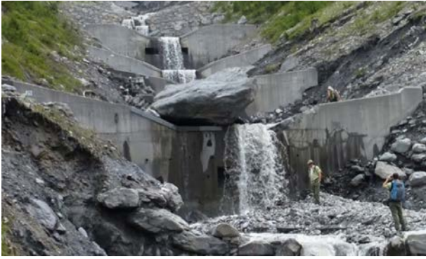
Figure 1.9 – Huge boulder stopped on the check dam series of the St. Antoine torrent upper basin (73 – FRA.) – 2014 (photo courtesy of S. Carladous)
