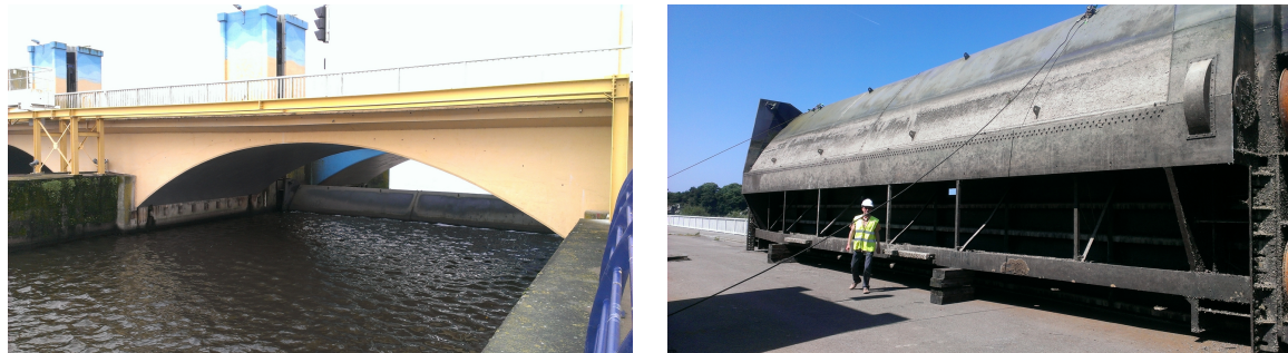
Figure 6.3: Pictures of a shutter in operation (left) and a shutter and upper gate taken out of the dam for maintenance (right).
