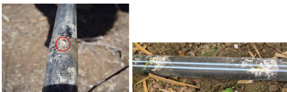
Figure I.8: Chemical clogging observed at the output of a conduct orifice (example of clogging by precipitation of \text{CaCO}_3 ) (source: PReSTI)
