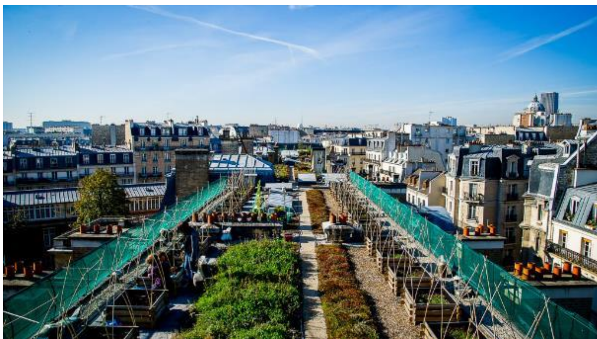
Figure 95 : The rooftop of AgroParisTech in 2012. On the right side the first crop sequence (experimental device n°1) (Photo credit: Xavier Remongin)
