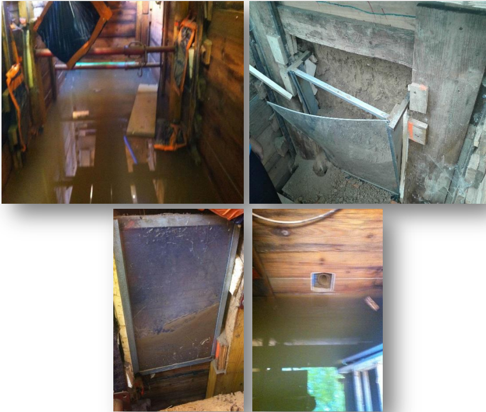
Appendix. 4: Flood damages
