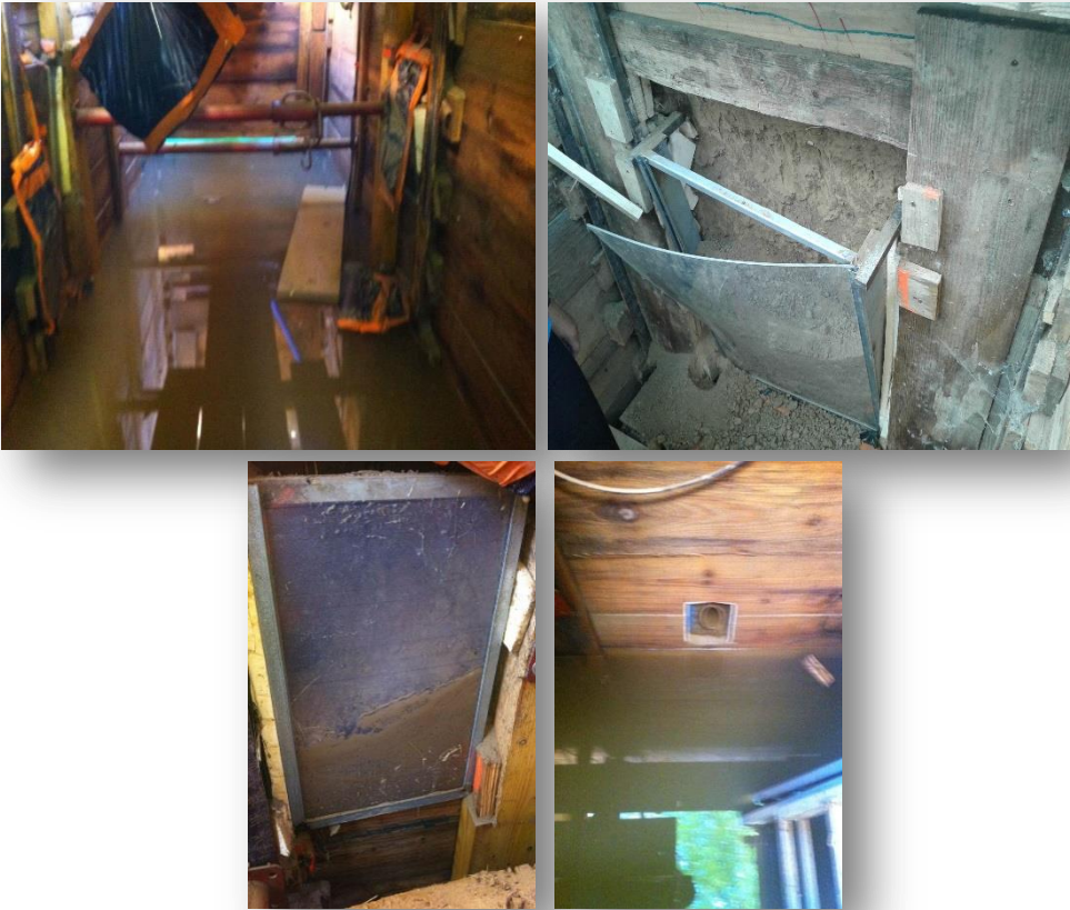
Appendix. 4: Flood damages
