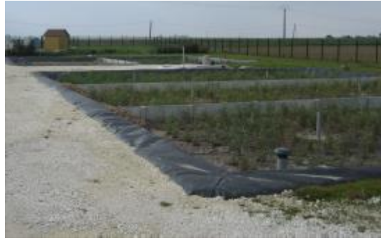
Filters planted with reeds (Cemeux, 250 PE)
