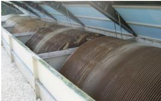
Rotating biological contactor (Saints, 900 PE)
