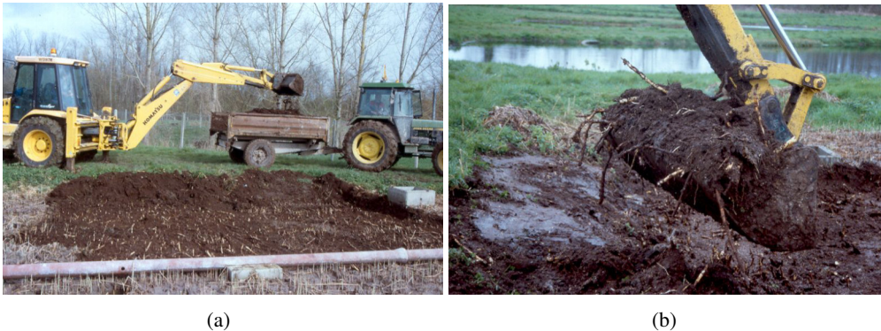
Figure 2.45: Dredging of the deposit layer in French VFTW
