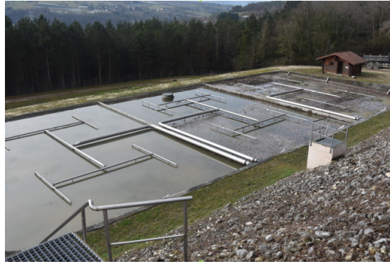
Figure 2.8: Clogged 1st stage in Copponex TW (Haute-Savoie, France, 2016).
